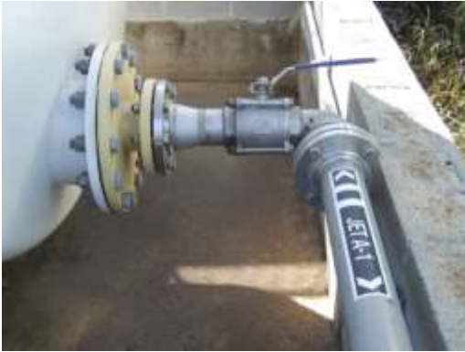
MAIN FUEL SUPPLY SHUT OFF VALVE
