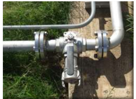
"T" PORT FUEL SHUT OFF/DIVERSION VALVE AND ALTERNATE FUEL PICKUP FROM TANK VALVE
